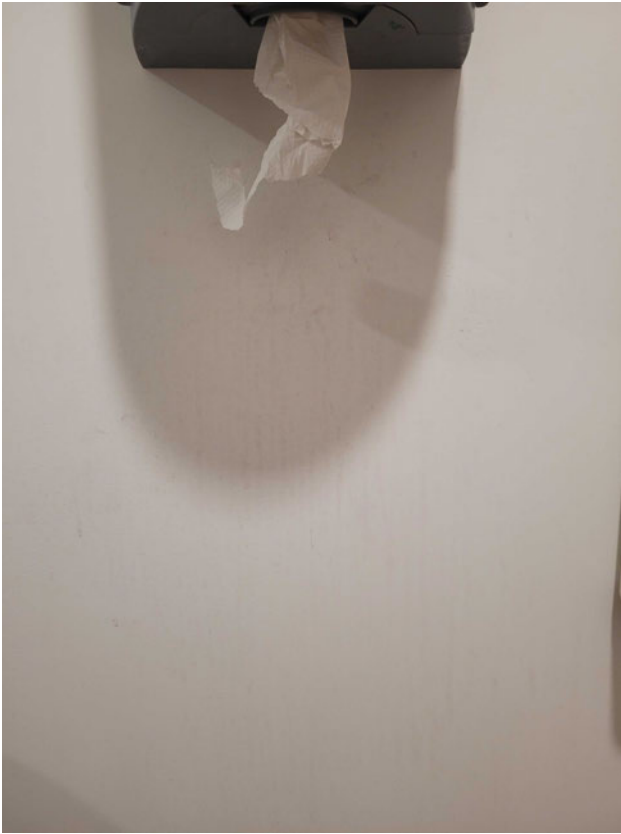
Wall by upstairs bathroom paper towel dispenser. Streaks go all the way to the floor.
