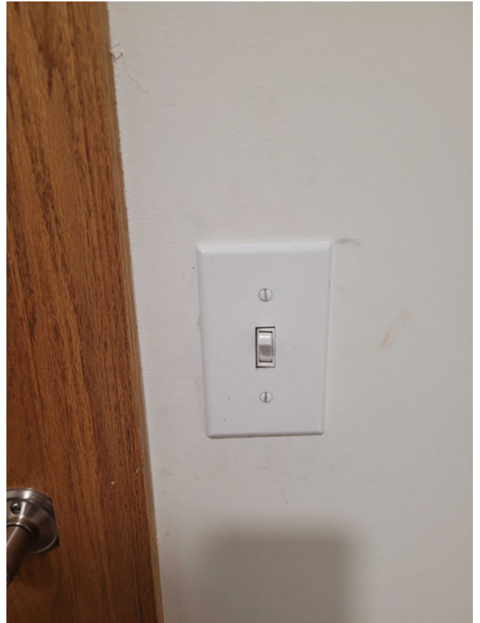
Wall by upstairs bathroom light switch
