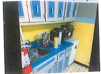
These cabinet doors and frame included; no interior of cabinet
